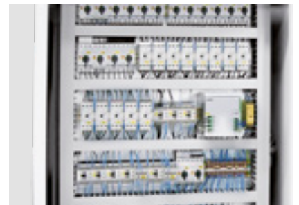
Freestanding switch cabinet with cooling unit and separate frequency converter per motor
